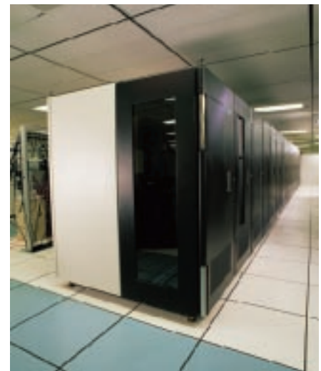
A Magstar 3494 tape library 16-frame high-availability configuration with two service bay frames.
