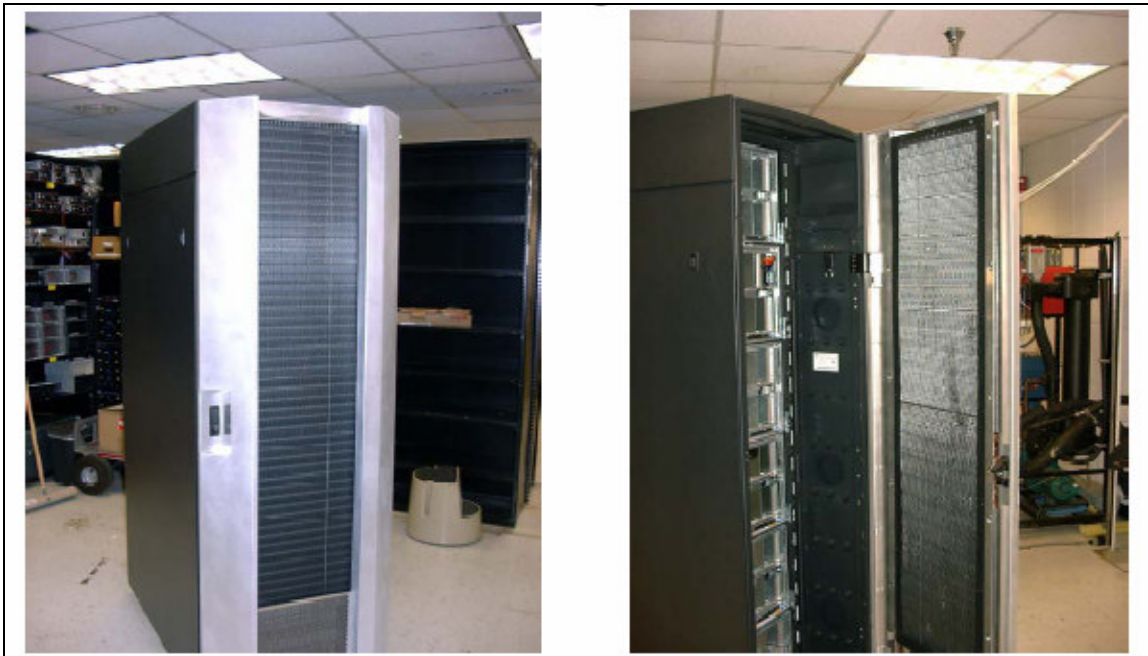
Figure 5. IBM Rear Door Heat eXchanger with door closed (L.) and open (R.)
